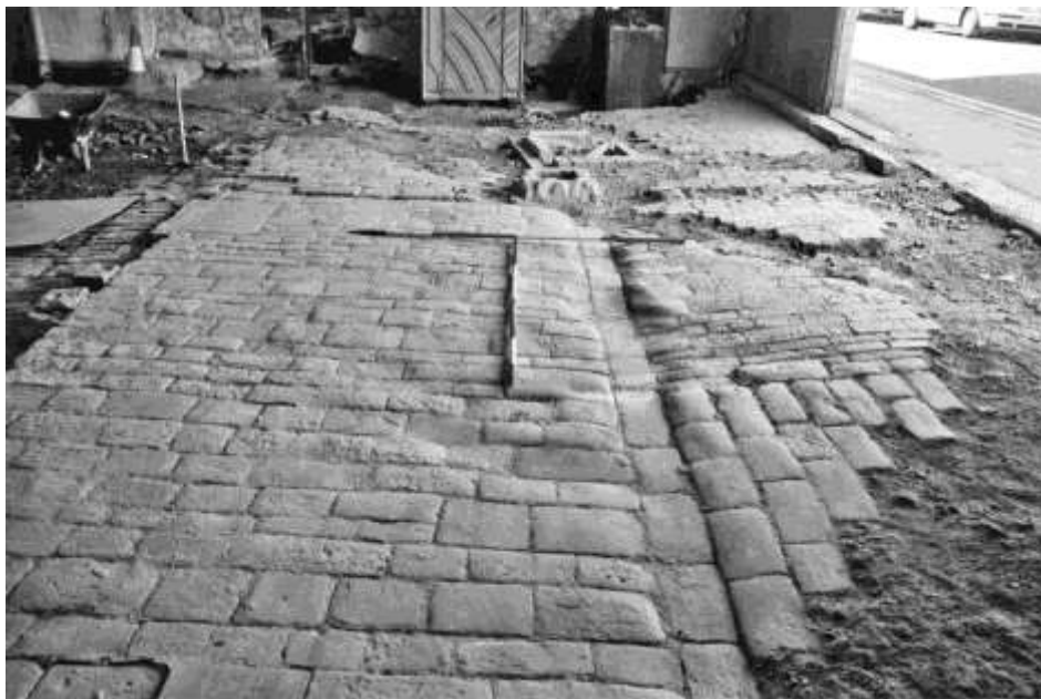
Front yard. Note the wear pattern showing where coaches turned in front of the door and front wall, left
